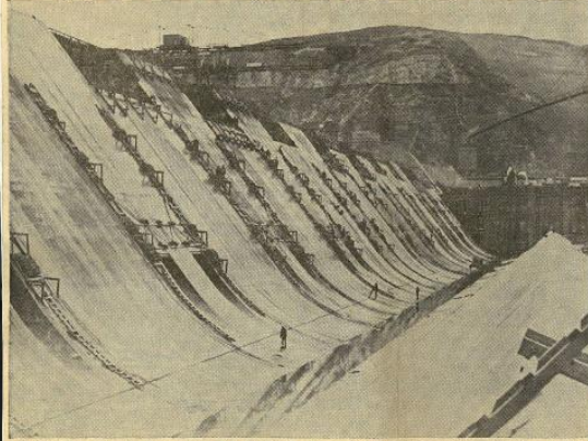
On the downstream side of the massive concrete barrier which has been erected across the original bed of the Columbia river a mammoth trough has been constructed to break the force of the cascade which will surge over the spillway when the Grand Coulee dam is completed. The picture at the left shows the scene Wednesday just before the timber cofferdam was opened to permit the waters to fill the east side pit, preparatory to turning the Columbia back into its old channel.
