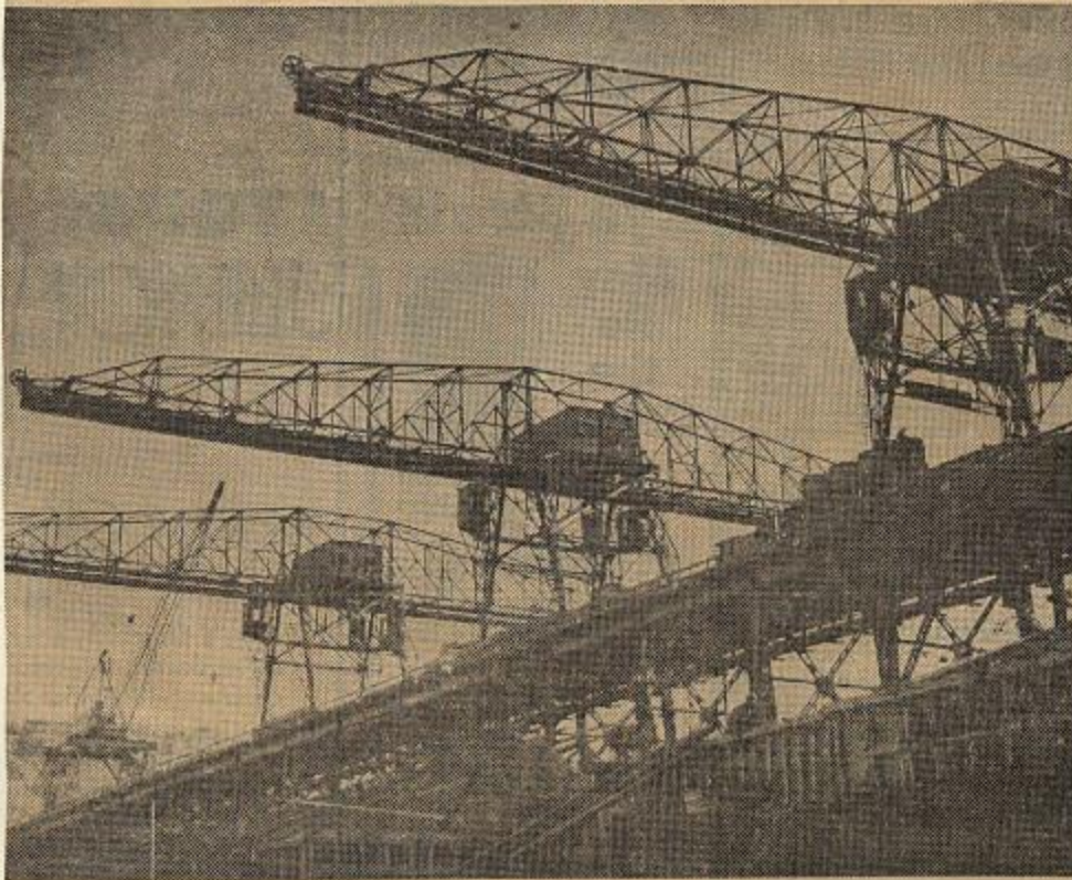
Hammerhead cranes on the trestle from which concrete is placed in the Grand Coulee dam, under construction by the bureau of reclamation on the Columbia river in eastern Washington. This equipment has placed a maximum of more than 8000 cubic yards of concrete a day. About 1,750,000 cubic yards of concrete has been placed in the west section of the dam. Note that the forms here are approaching the maximum height of the placing trestle.
